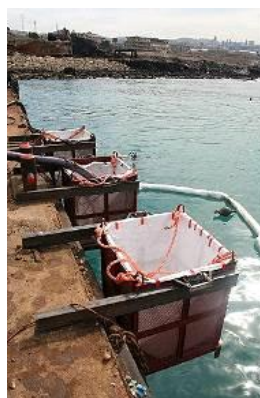
Figure 30. Filtering system to separate sediment/oil from the water utilised
